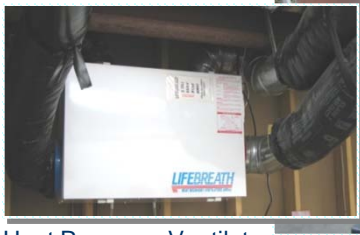
Heat Recovery Ventilator
